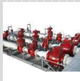
Pressure reducing stations
